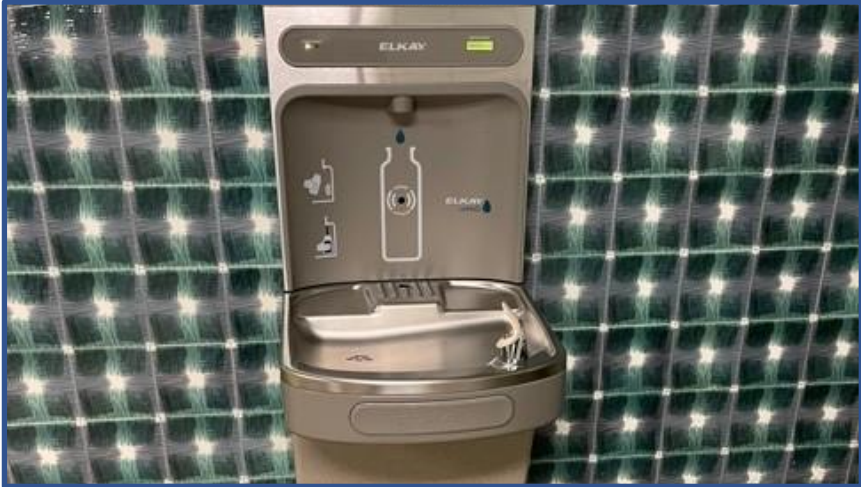
Water filling stations at Gregorian
